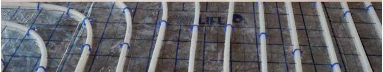
HEALTHY HYDRONIC SURFACE HEATING
